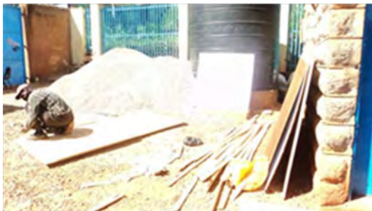
Some of the construction materials and carpenter at work doing some renovations which are normally
